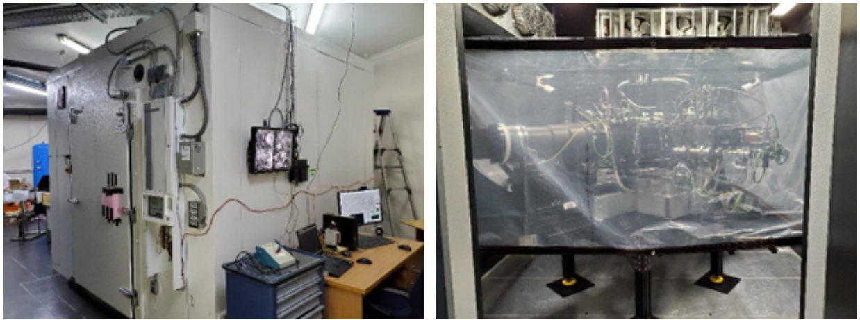
Figure 1. The NIR enclosure in the SALT Spectrometer Room (left) and the instrument inside (right). The fiber cable will enter the enclosure through the rectangular hole (currently filled with pink foam) in the upper left corner above the door. The plastic shroud around the spectrograph is to shield optical components from direct air currents from the cooling system.
